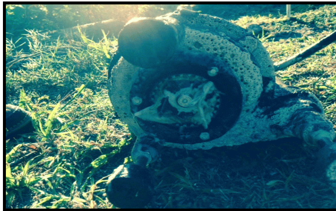
Lift Station Pump Clogged with Wipes
